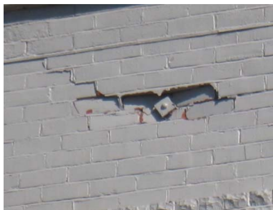
Fig. 23 Close up of partial anchorage failure. Photograph of damage in the 2010 Darfield (Canterbury) earthquake due to deficient anchorages [Ingham, 2012]
