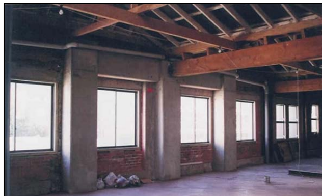
Fig. 32 A concrete moment frame inside the façade of a large URM building in Wellington (Dunning Thornton Consultants)
