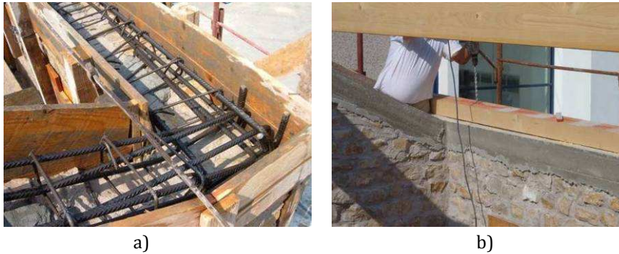
Fig. 30 Details of the reinforcement of the ring beam (left) and view of the ring beam after filling with the concrete (right) [Magenes et al, 2012]
