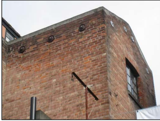
Fig. 24 Successful anchorages spaced close together. Photograph of building after the 2010 Darfield (Canterbury) earthquake [Ingham, 2012]
