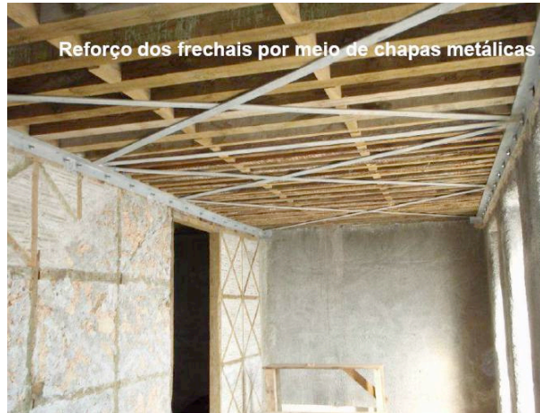
Fig. 13 In-plane stiffening with metallic diagonals and reinforcement of connection floor-wall (Pombalino building) [photo from Edifer]
