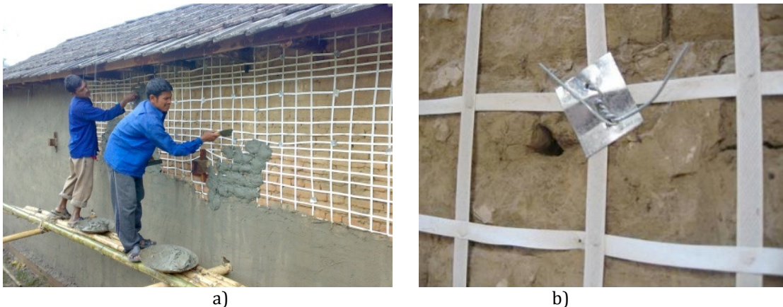
Fig. 11 Implementation of PP band method of retrofitting in Kathmandu Valley (a) and anchorage throughout the wall (b) [Shrestha et al. 2012]
