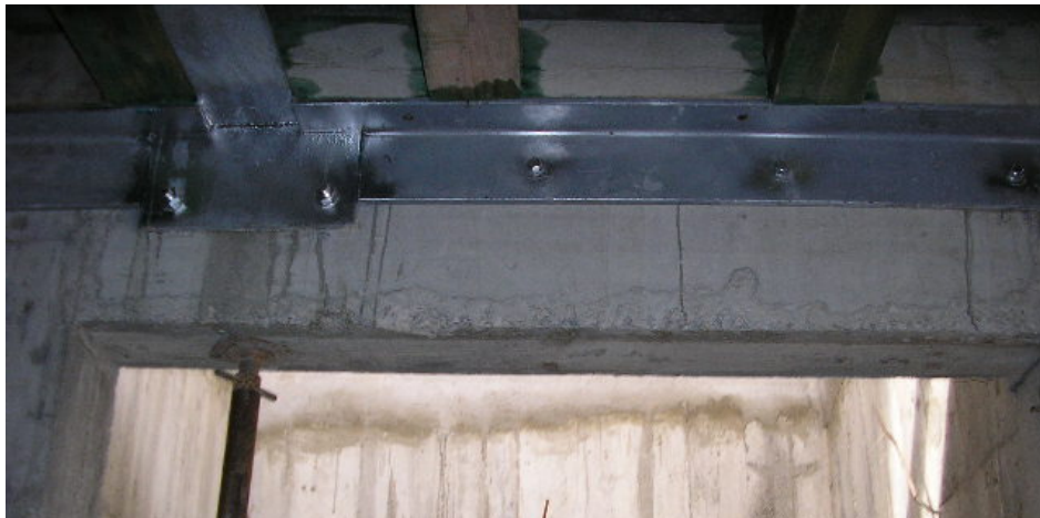
Fig. 14 Photo of the connection with L-shaped steel plates between wooden floor and masonry wall
