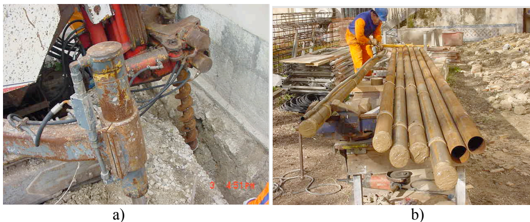
Fig. 5 a) Machine to drill the holes, b) micro piles casing to be filled with cement grout [photos by Appleton, 2011]
