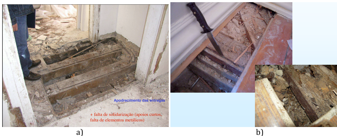
Fig. 9 a) Rotten wood joists at the connection to the wall; b) Rotten wood elements [Cruz, 2012]
