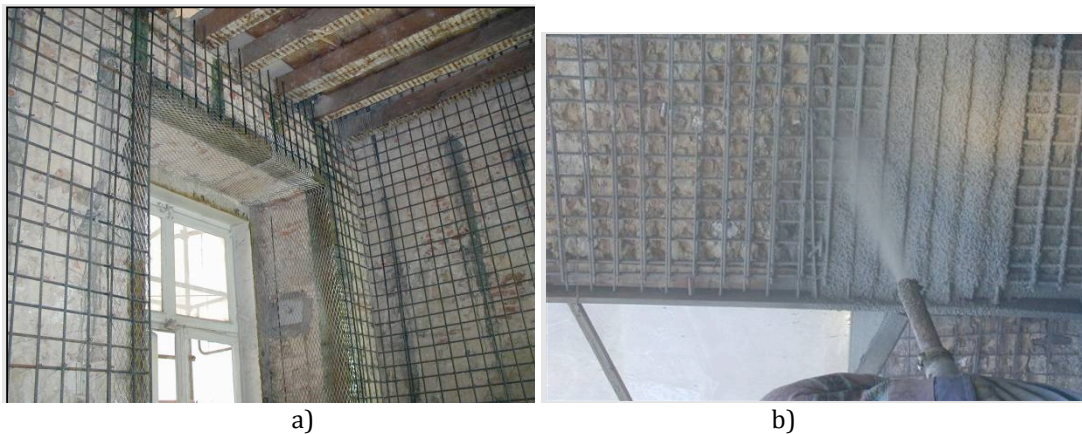
Fig. 10 a) Masonry wall from the inside with steel mesh, b) spraying of the cement grout into the wall [fotos by Appleton, 2011]
