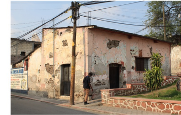
Grade 2: Moderate damage (slight structural damage, moderate non-structural damage).
