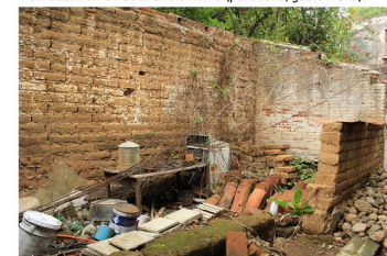
Grade 5: Destruction (very heavy structural damage)
