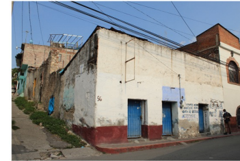
Grade 1: Negligible to slight damage (no structural damage, slight non-structural damage).
