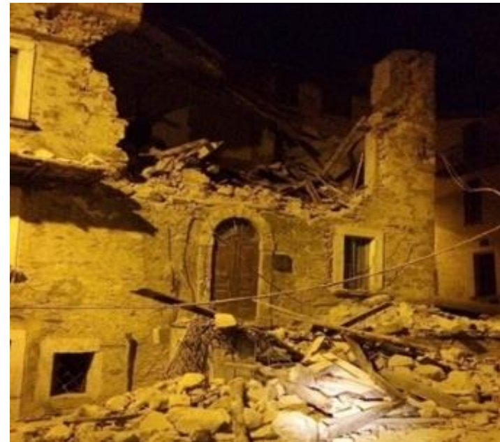
Out-of-plane failure mechanism
