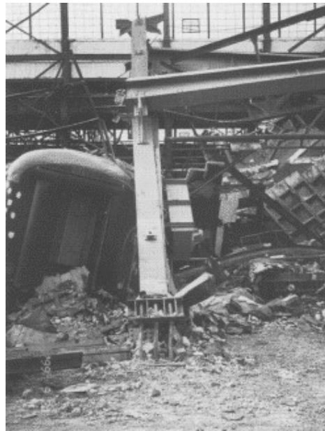
Figure 1 – Damages at Turkiye Vagon Sanayii A.S. factory in Adapazari
