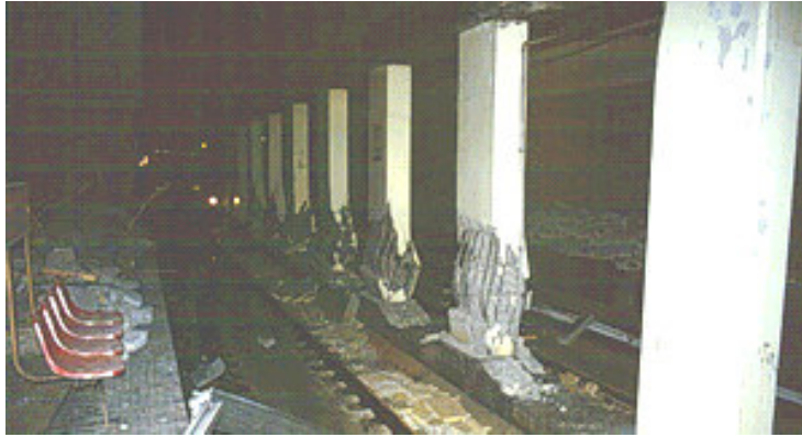
Figure 2.1. Collapse of the central columns of Dakai tube station, Kobe, Japan
